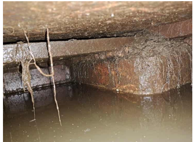
Figure 5 - Chamber wall 1 RHS 1.1 – wall is resting on this lintel and concrete cover
