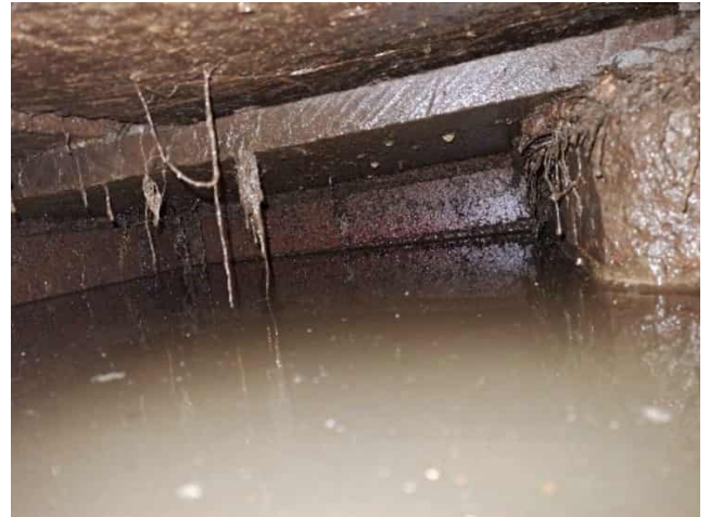
Figure 4 - Chamber wall 1 RHS 1.0 – wall is resting on this lintel and concrete cover
